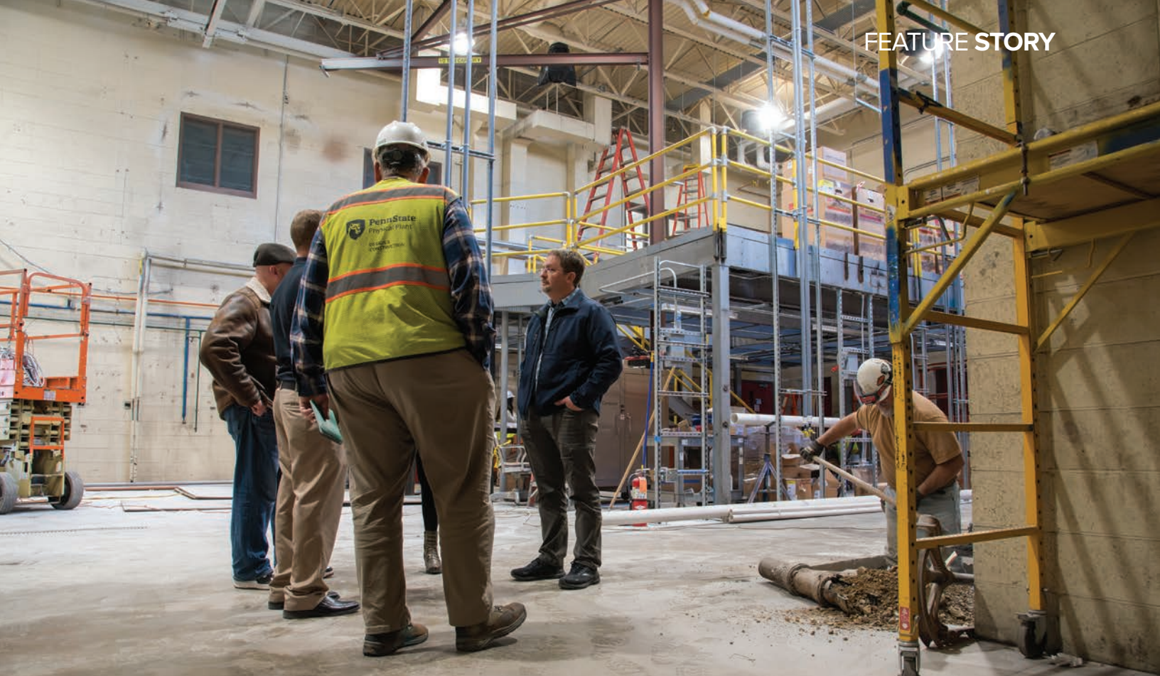
Robinson, center, oversees the creation of the new 2,400-square-foot SiC research facility at University Park.
